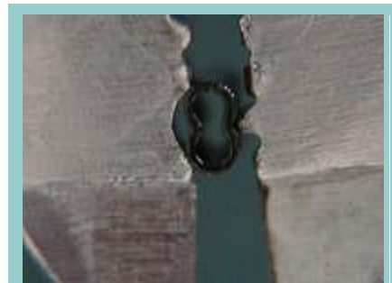
Using the wrong tool will cause the joint to fail under pressure
